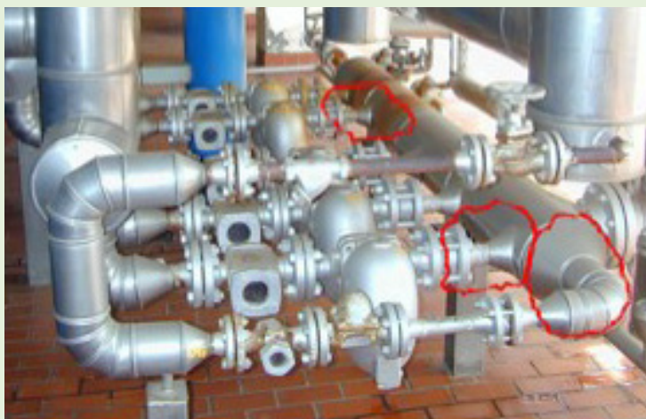
Steam Trap Installation
