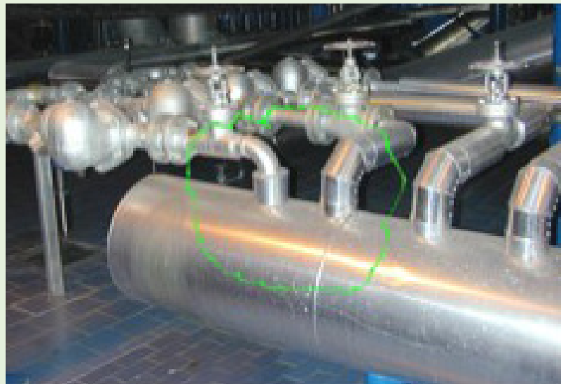
Picture indicates the proper connections to the main condensate header
