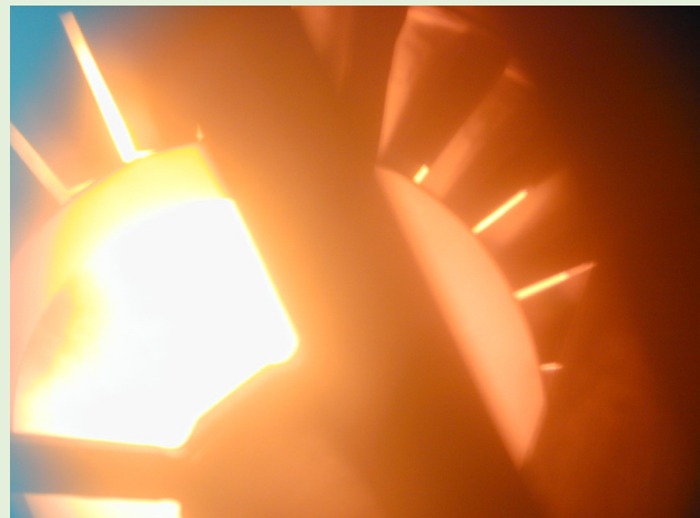
Natural Gas-Fired Burner
