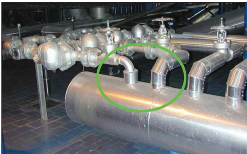
FIGURE 5. The green circle indicates the proper connections to the main condensate header
