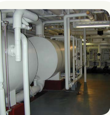
Condensate tank totally insulated
