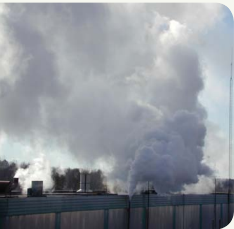
Steam blowing to atmosphere - A loss of steam and condensate
